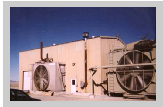
Central Compressor Facility
