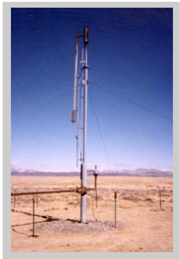
Waste Gas Flare Tower
