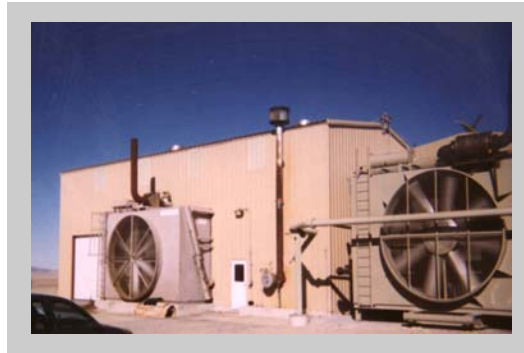
Central Compressor Facility
