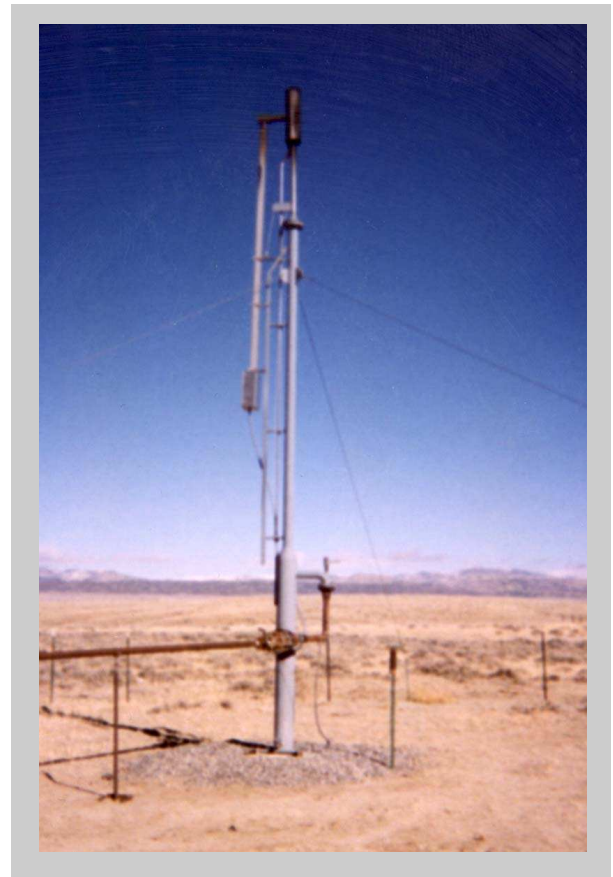
Waste Gas Flare Tower
