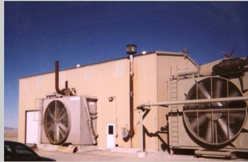
Central Compressor Facility
