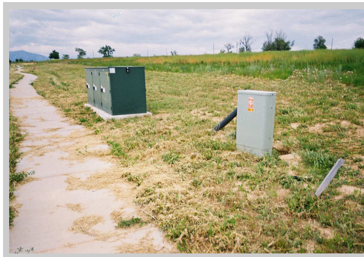
Undeveloped property with a transformer
