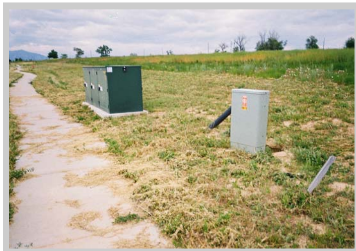
Undeveloped property with a transformer
