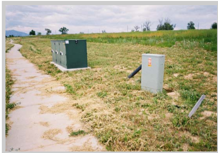
Undeveloped property with a transformer
